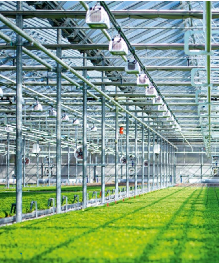
The helioCORE control system and dimmable luminaires supplement the daylight that flows in through greenhouse glazing automatically with the right quantity of electric light.
